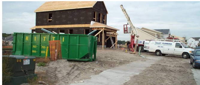
Photo caption: Construction practices can result in significant soil compaction. (Image Source: All photos in this document taken by Fred Rozumalski)
