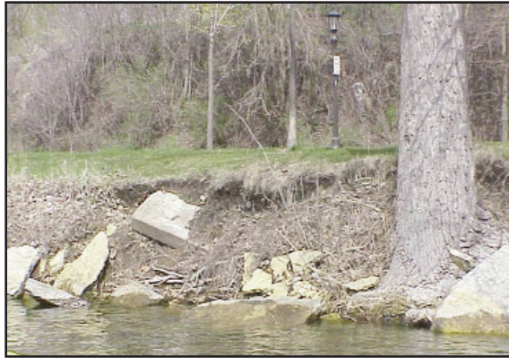
Figure 3. A typical stretch of eroded shore - 1999.
