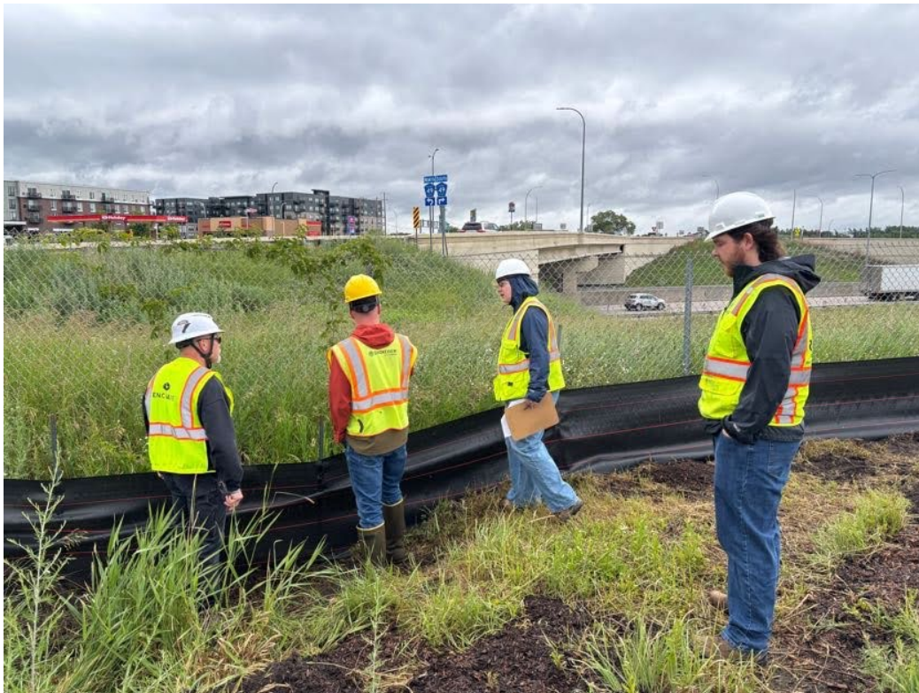
RWMWD staff inspecting silt fence installation with City of Shoreview and contractor staff at Permit site #24-34 Rice Street Crossings (Krew Apartments) off I-694 and Rice Street
