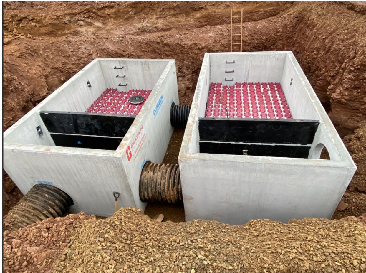
Figure 3-2 Large underground Jellyfish Filter systems (Contech Engineering Solutions, 2026)
