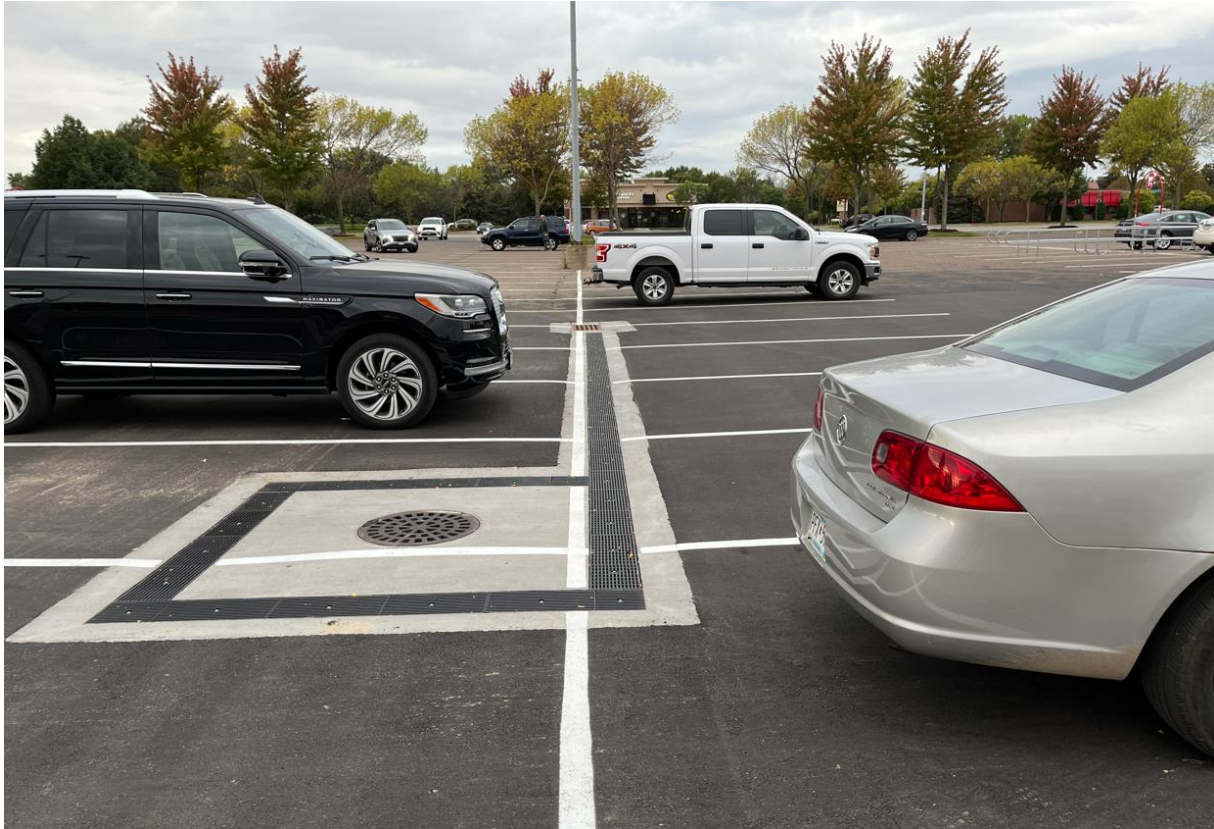
Figure 2: The completed trench drains that will collect runoff in the north parking lot and direct to the north filtration rain garden for treatment
