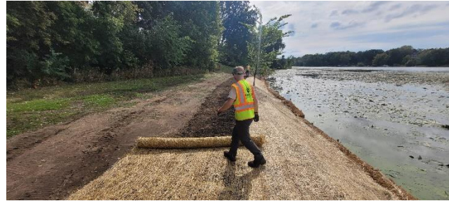
Keller Shore Phase 2 Install- top to bottom: Installing biologs, jetting in rock, rolling out erosion control fabric.
