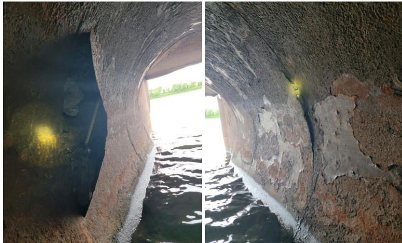
Figure-2 Deformation and joint separations in nine-foot-diameter steel pipe
