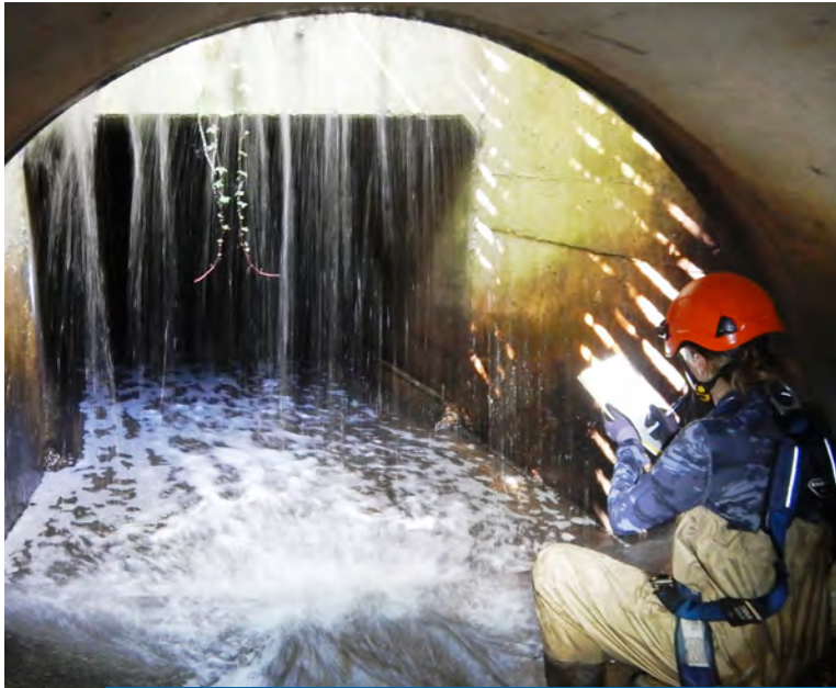
Installation of the Battle Creek tunnel was one of the RWMWD's first projects in the late 1970s and early 1980s. Barr helped the district with the original study, design, and installation coordination. We continue to assist with monitoring, inspection, and design as well as oversight of maintenance work to enable the over one-mile-long tunnel to continue to convey flows from southern portions of Saint Paul and Maplewood as well as from Oakdale and Woodbury to the Mississippi River.
