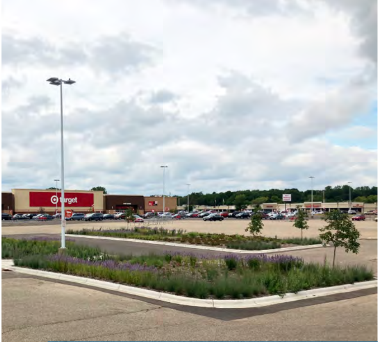
Over the past few years, Barr has assisted the RWMWD in the design and implementation of stormwater retrofit and green infrastructure features at two Saint Paul Target stores and a third store in Woodbury. The projects included removal of impervious parking spaces, installation of infiltration rain gardens, and construction of tree trenches. This photo shows two rain gardens constructed in the parking lot of the North Saint Paul Target site.
