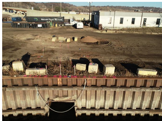
Above: Drone photo of where the Beltline tunnel meets the Mississippi River through a river wall owned by Saint Paul Port Authority. The concrete blocks in the background show the manhole location, which is the upstream limit of the proposed tunnel replacement.
