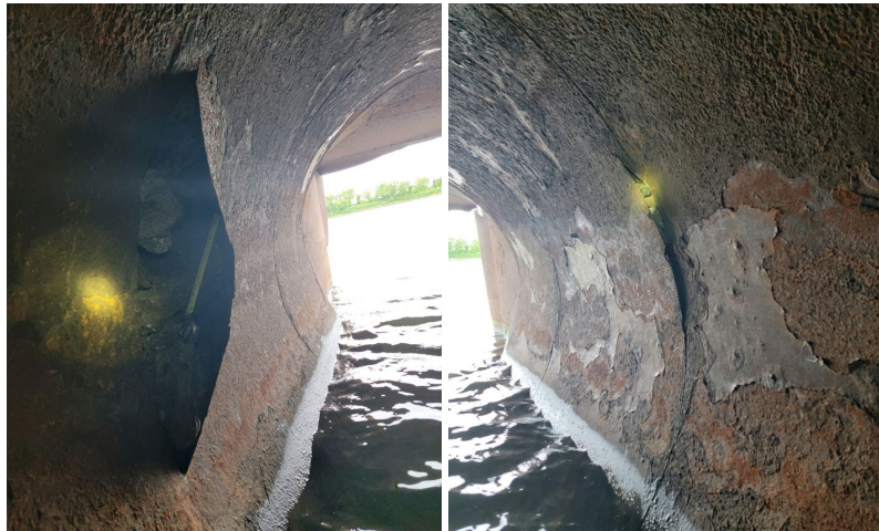
Figure 1-2 Deformation and joint separations in nine-foot-diameter steel pipe
