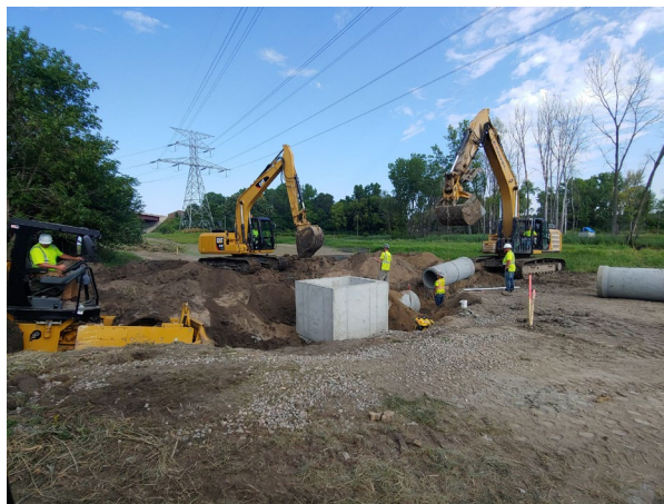
August 21, 2020, facing northwest: The MnDOT pond is to the left (not shown). The concrete box is the manhole where the dropdown weir and backflow preventer will be located. The contractor is shown backfilling and compacting the pipe.
