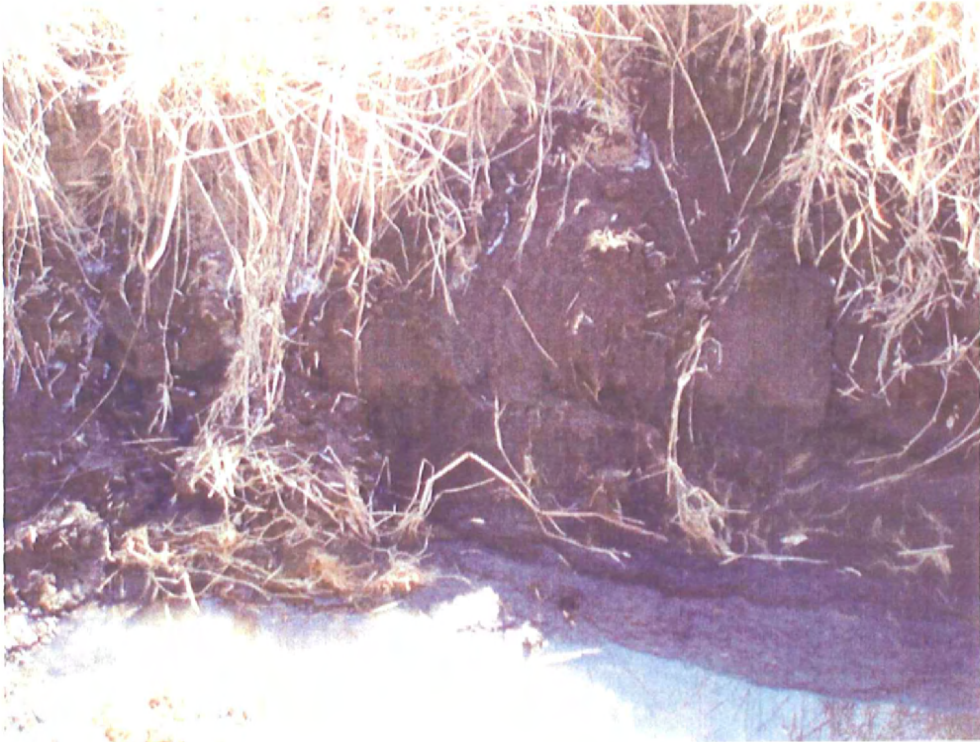
Stream bank erosion in the upstream portion of the creek near the outlet from Bailey wetland
