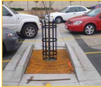
Completed tree trench with concrete swale and curb and tree cage to protect trees from cars.
