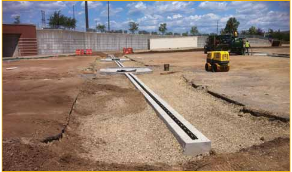
Tree trench with trench drain rather than swale. This trench has the class 5 installed, ready for new asphalt.
