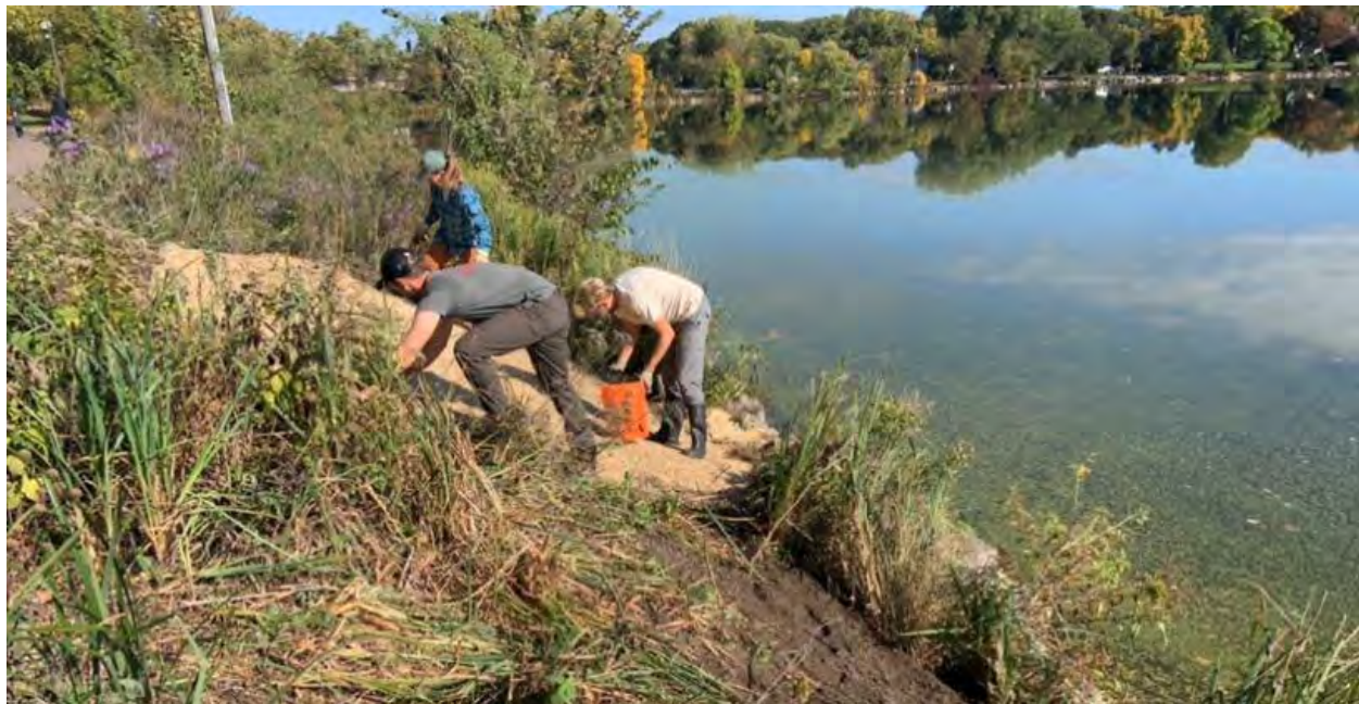
A short grass prairie seed mix was spread on the slope and then covered with a degradable erosion control blanket. Plant plugs were then planted through the blanket.
