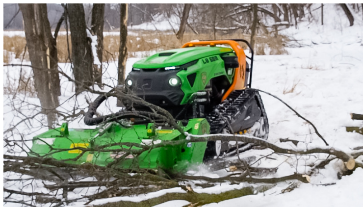
The green climber was used to cut and mulch dead tree and buckthorn branches. This opened up the shoreline for the wetland edge planting that will take place in summer 2020.
