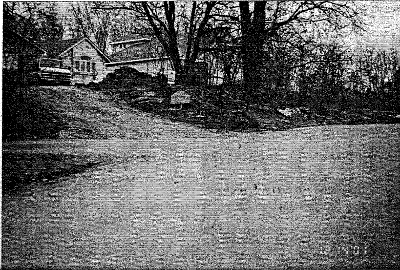
Photo of residential construction site on White Bear Ave. near "C" Street with no erosion control practices being used.
