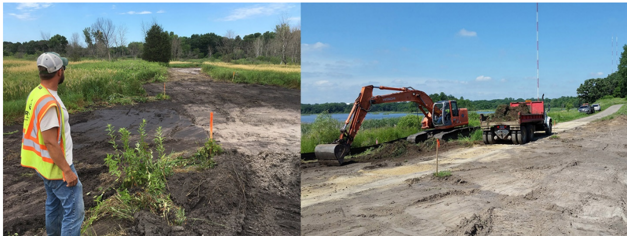
Water Quality Technician Dave Vlasin looks over a constructed wetland (left) designed to accept water from Grass Lake’s new overflow path (right).
