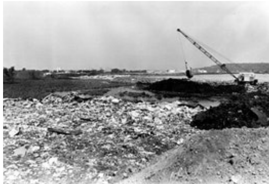
The sprawling 200-acre Pig's Eye Municipal Landfill on St. Paul's far south side in 1967. Photo credit William Seaman, RPA - Minneapolis Star Tribune
